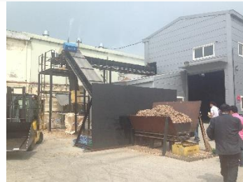
Fuels supply (Belt conveyer )
