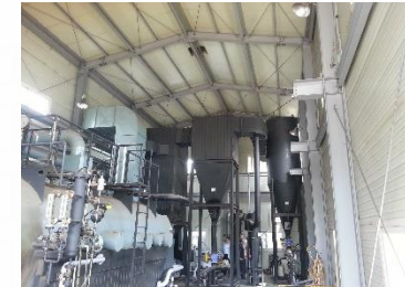
Bio energy steam supply system
