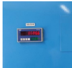
Boiler steam flowmeter
