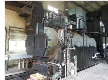
Automatic biomass water spray complex boiler
