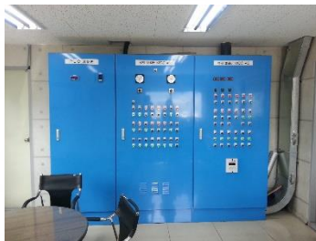
Electric control (PLC MCC )
